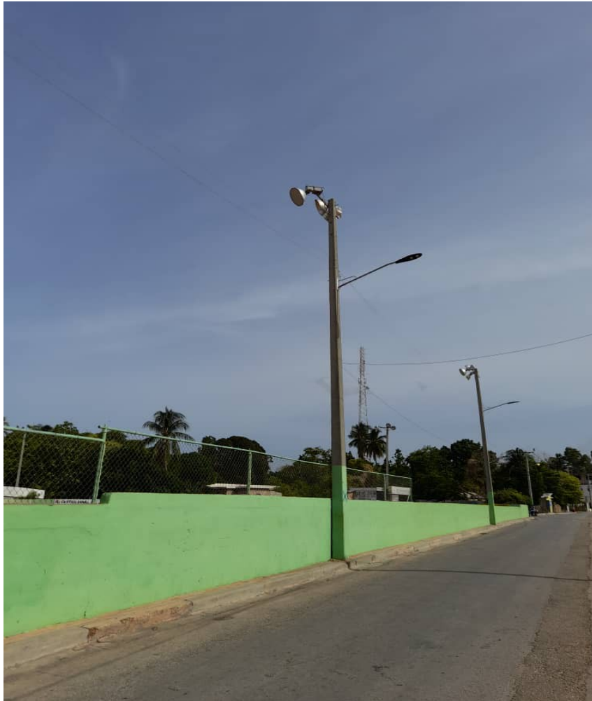
Photo 13: Light system of baseball stadium
