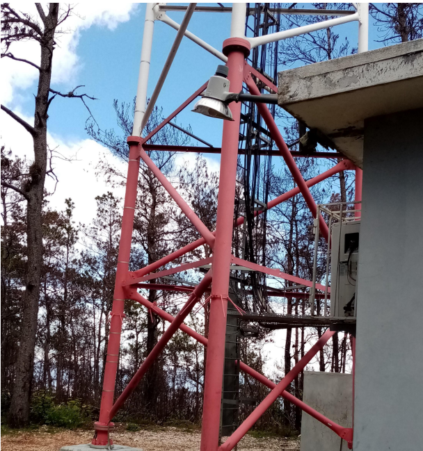
Photo 5. Altice tower security light
