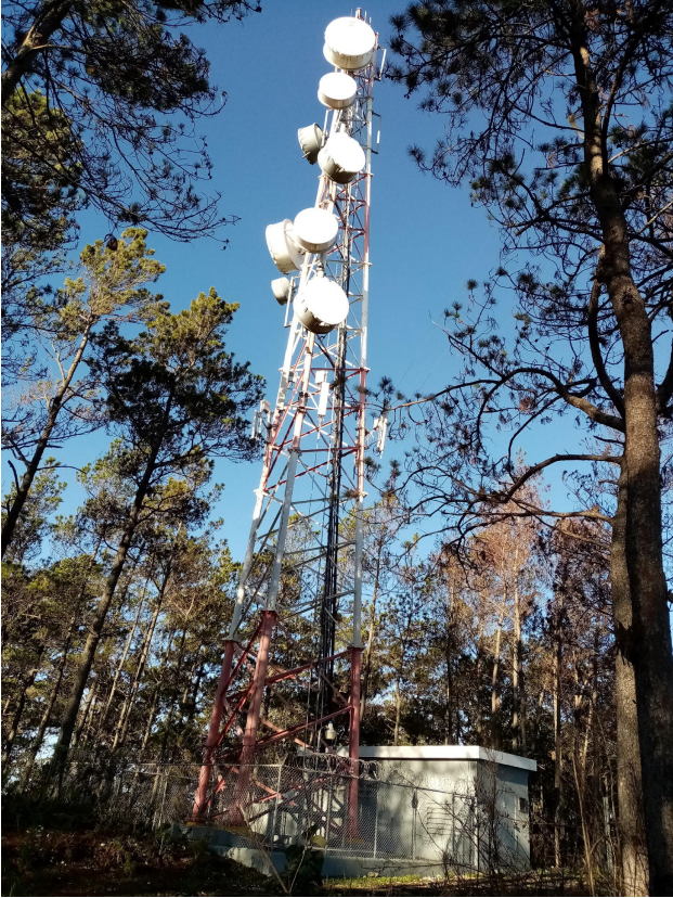
Photo 2: Claro communication tower
