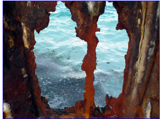
Rusting sheet metal piling
