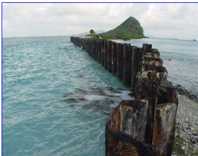
Sheet metal piling and causeway restricting the flow of water into the lagoon near Frigate Island
